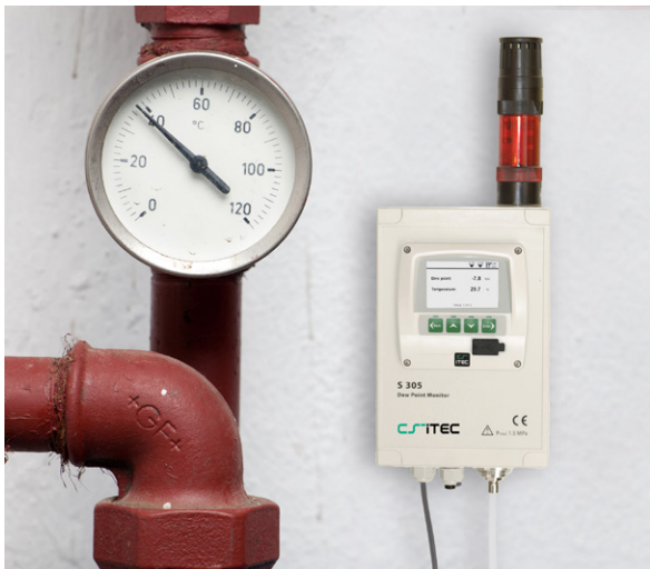
Alarm adjustment at dew point sensor
